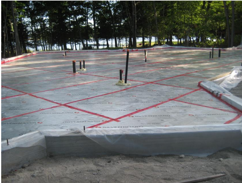
7. Foundation/Grid of heated floors
