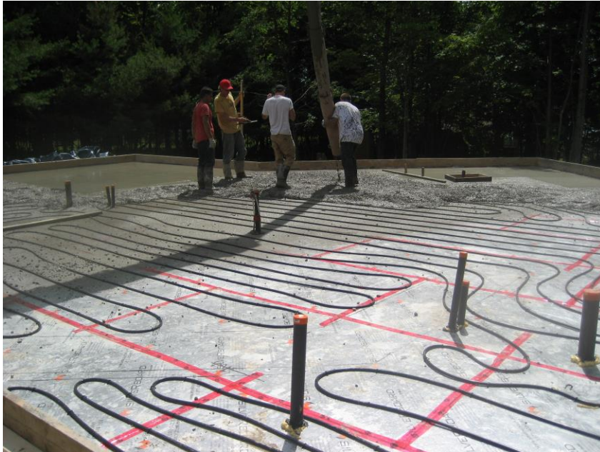
5. Heated Floor Tubing
