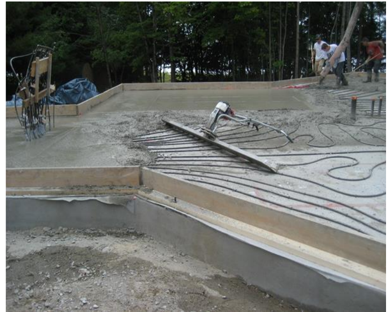
4. Heated Floor Tubing
