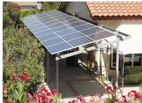
Solar Panels on breezeway
