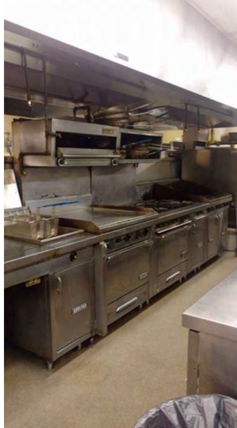
Ovens and Burners
